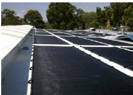
Solar pool heating system on the roof of Belmont Oasis Leisure Centre
