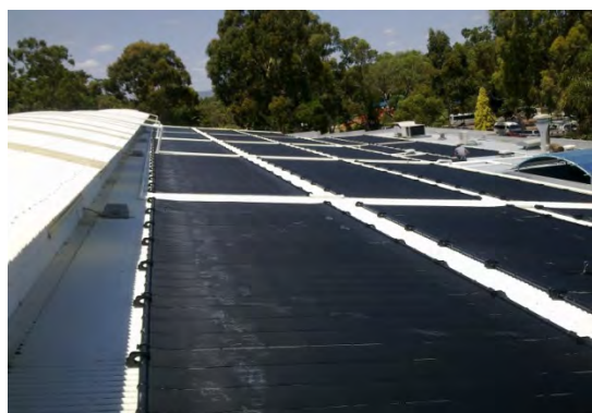
Solar pool heating system on the roof of Belmont Oasis Leisure Centre
