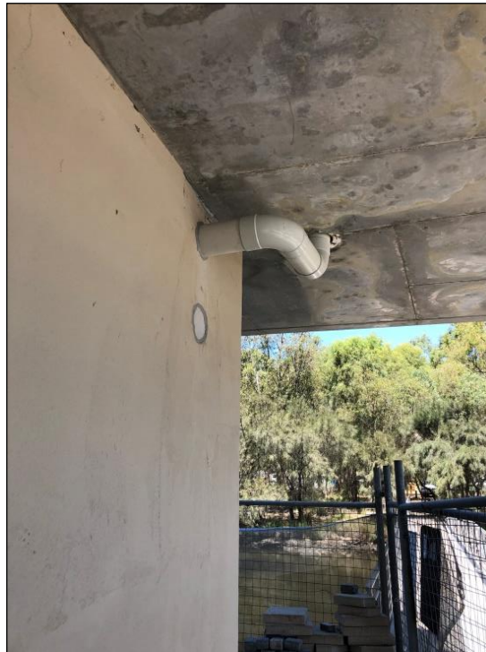
Figure 4: Minor drainage pipe encroachment
